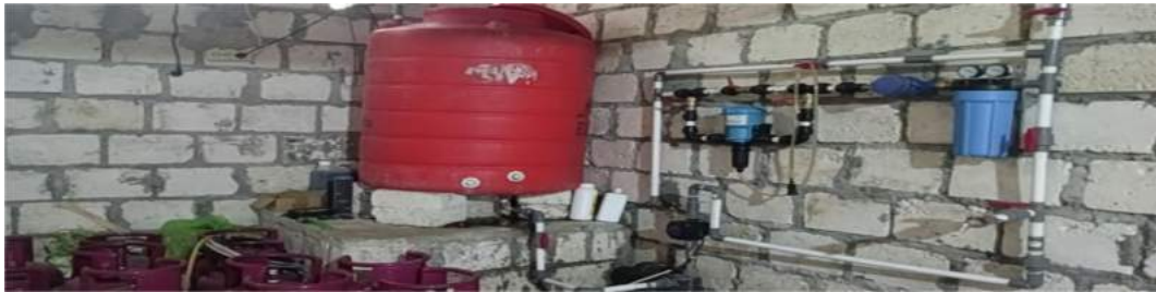
Gambar 10. Instalasi Air Kandang CH. Hj. Gusmiati
