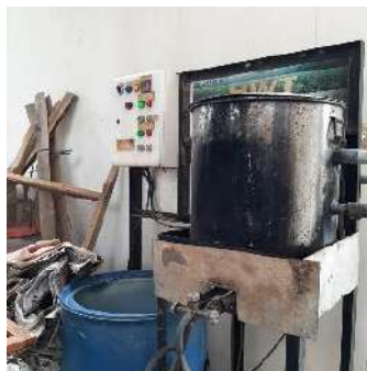
Gambar 4.4 Tangki hot water treatment
