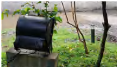
Figure 5. Flood lighting directed to river stream.
