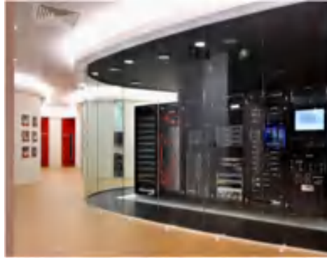
Figure 4. Server room, on-premises data storage. Source: pinterest
